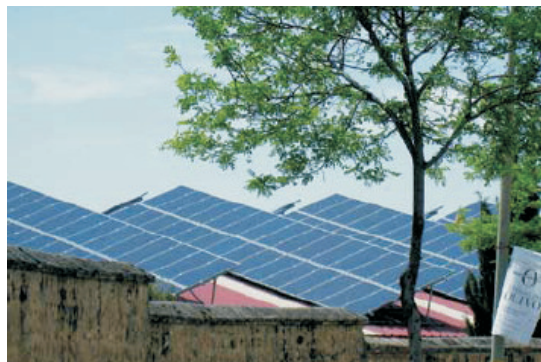
Solar panels on the roof of a sports stadium in the Spanish town of Baeza
