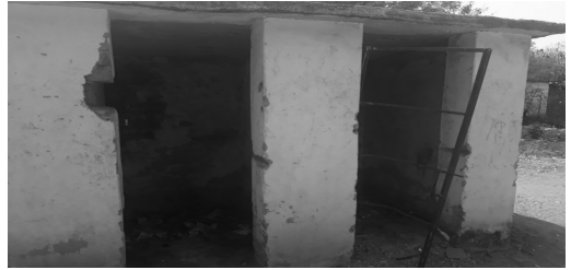
Figure 2. Toilets in Dilapidated Condition
